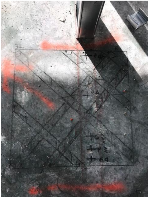
Scan #37/Denoted as 32: This scan shows an 8" slab with a top and bottom layer of rebar.
