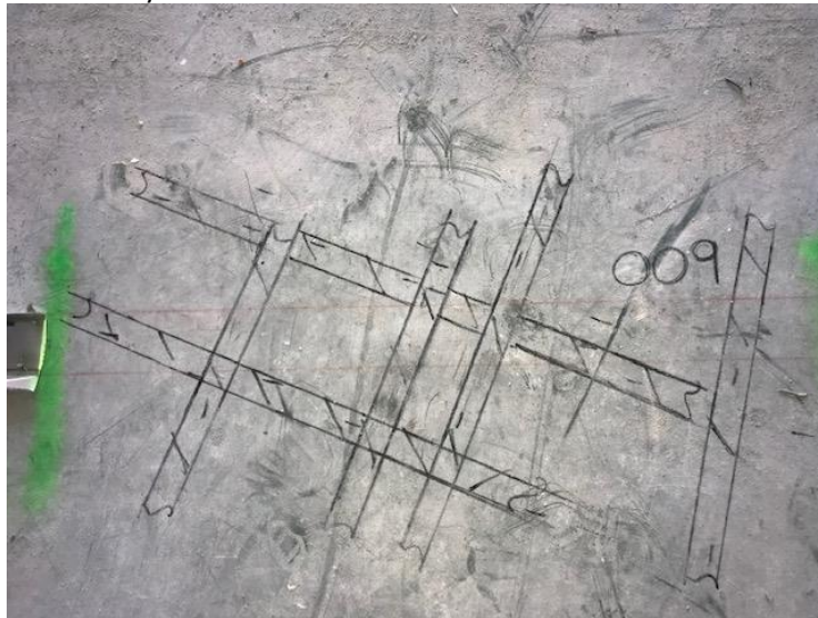
Scan #39/Denoted as 009: This scan shows an 8" slab with a bottom layer of rebar.
